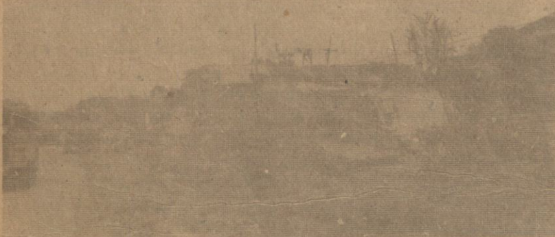
The demolished structures ready to be hauled to the relocation site at the Tala estate of the NHA in Novaliches.
