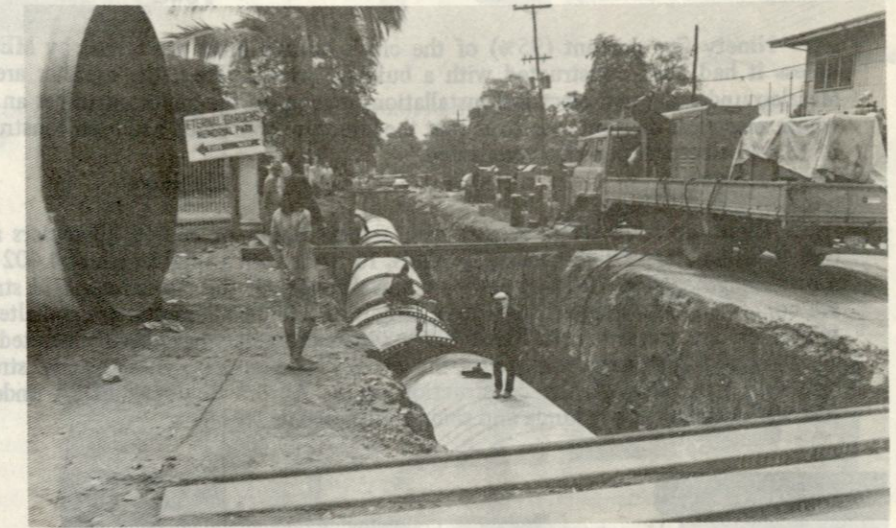
Last May 12, the First Lady and Mayor Rodriguez inaugurated the first phase of the Novaliches Waterworks which involved the laying of 35 kms. of water pipelines such as shown at right. The second phase is due for completion in May next year involving 40 kms. more water pipelines.
