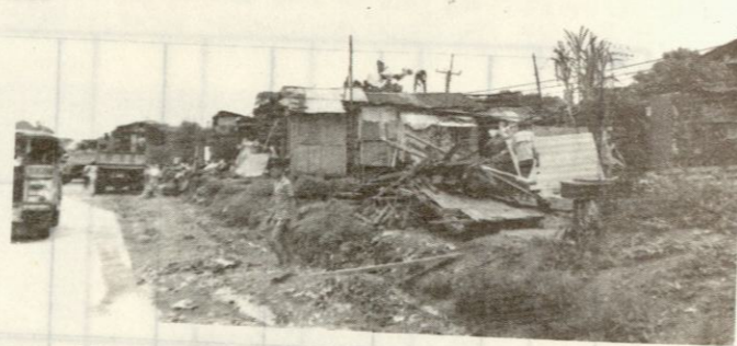
The dismantled structures are ready to be hauled by trucks to the relocation site at the Tala Estate in Novaliches.
