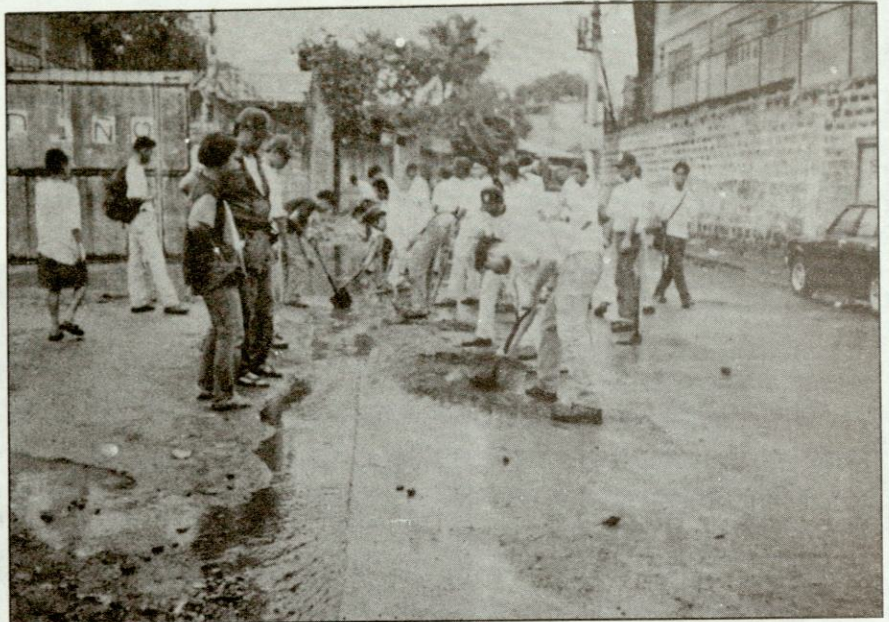
CAPT. DIÑO personally leads the asphalt patching in the city streets of San Antonio.
